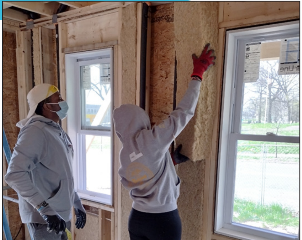
Students from Western New England University Pharmacy Degree program install Hempitecture HempWool at the Jackson Street, Holyoke, build site.
