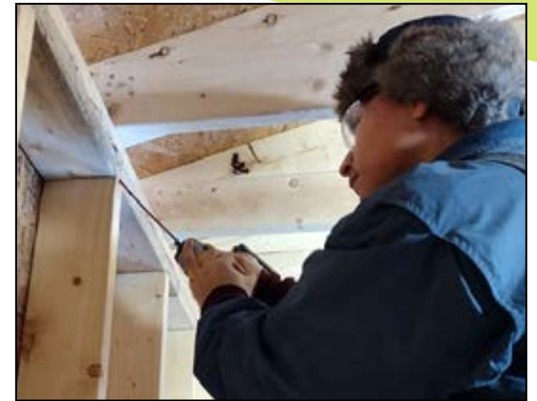
A carpentry student from Springfield's Roger L. Putnam Vocational Technical Academy works on the addition at Max's house.
