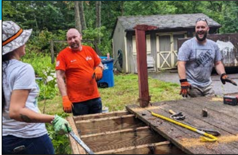
Volunteers from the Westfield Home Depot Distribution Center recently came out to Monson to help demolish a deck in preparation for a veteran repair project.
