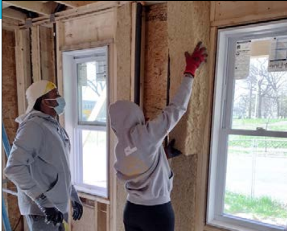
Students from Western New England University Pharmacy Degree program install Hempitecture HempWool at the Jackson Street, Holyoke, build site.
